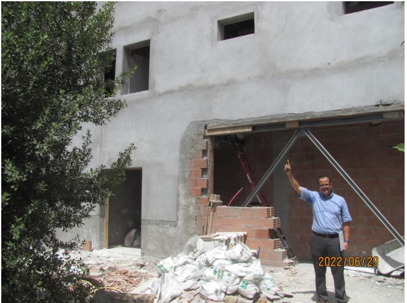
Here will be the brand new PASENSO centre in October 2022, Prof Laribi says.
